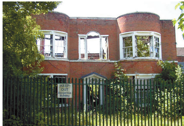
Mulberry Green after the fire damage
